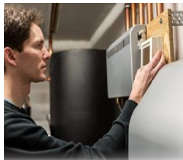
Biomass system heating control
